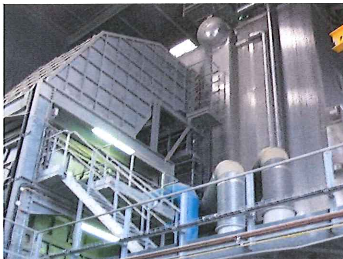
Post combustion - chaudière
